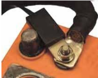
Fig 2.5(b) Temperature Sensor Installation
